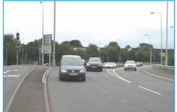
Cyclists leaving this roundabout can find themselves in the outside lane of a dual carriageway.
