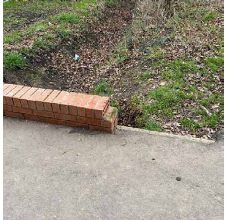
Image 2 Damaged wall and access to ditch
