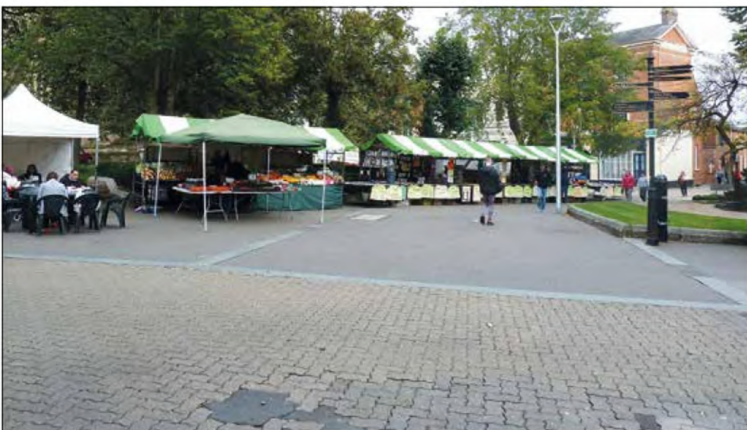
Patched block paving on Market Place
